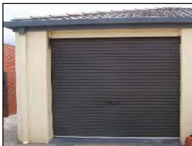
NON-COMPLIANT ROLLER DOOR
